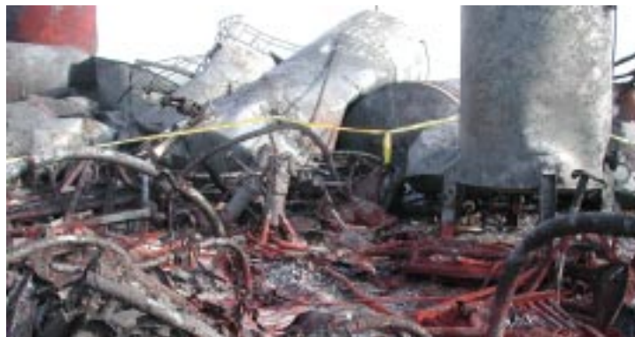
Figure 7. Collapsed blend tanks located near warehouse 1.
