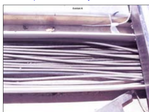
Fire at Mercantile Occupancy, California, April 2009
