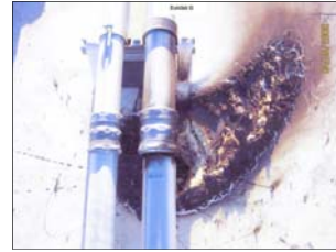
Fire at Mercantile Occupancy, California, April 2009
