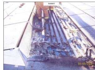
Fire at Mercantile Occupancy, California, April 2009
