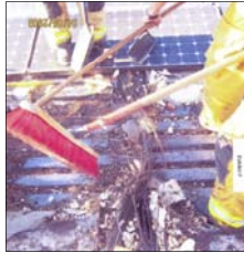
Fire at Mercantile Occupancy, California, April 2009
